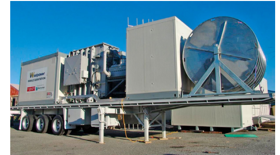
Spare mobile substation to speed up restoration
