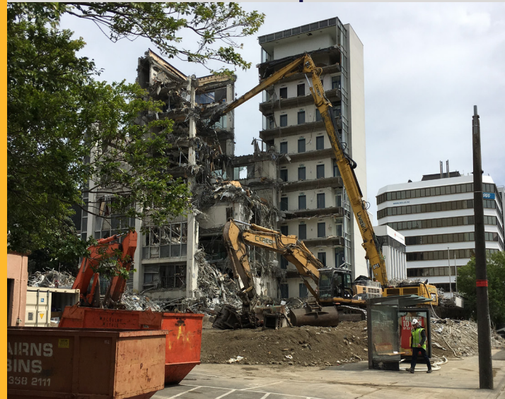
Post Kaikoura earthquake damage
